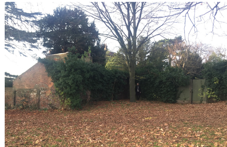
6. South End House boundary wall and gazebo with existing Stable Block fence
