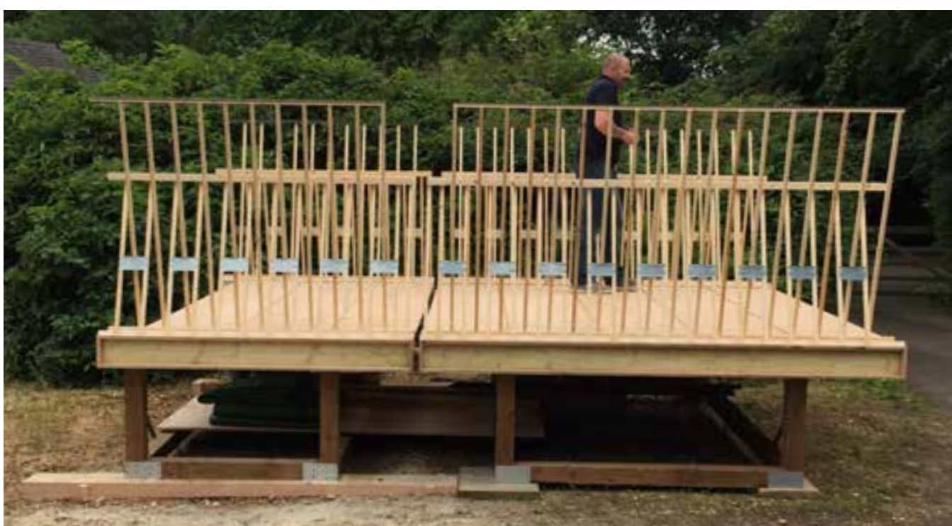
TRUE SCALE MOCK-UP MODEL OF BRIDGE CENTRE SECTION ( DESIGN TO BE AGREED)
